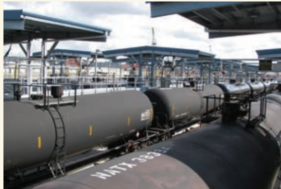
Rail loading facility.
