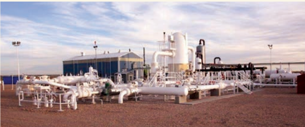
Natural gas compressor station.
