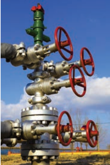
Natural gas wellhead.
