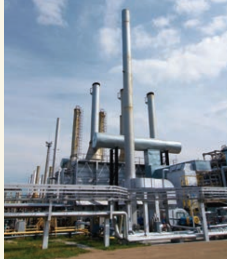
Natural gas processing facility.
