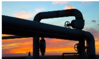
Interconnects with five interstate pipes and access to REX
